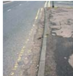
Grade D Heavily affected by detritus with significant accumulations
