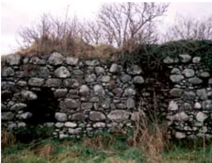
Tree roots can dislodge wall tops
