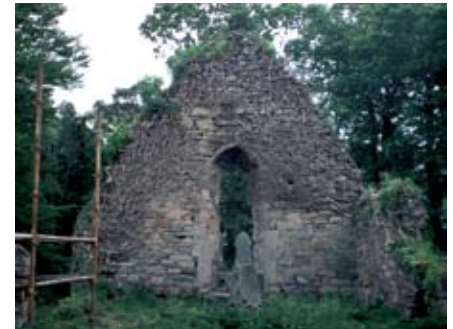
Elevation showing ivy after herbicide treatment
