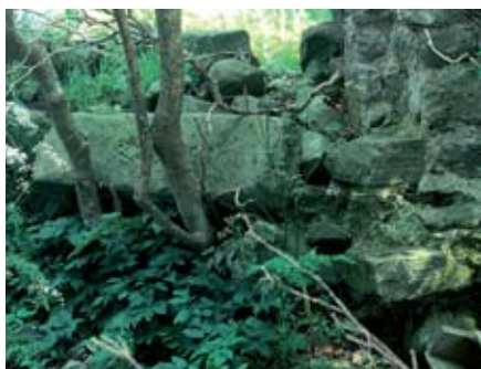
Displaced stones need to be recorded, removed & reset
