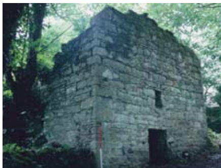
Mullycovet mill before repairs, Co. Fermanagh
