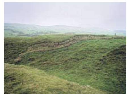
Sods were built up against the eroded face to conserve the earthwork
