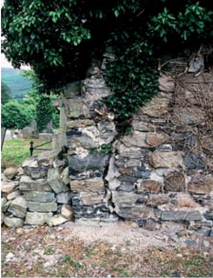
Damage to masonry by growing ivy
