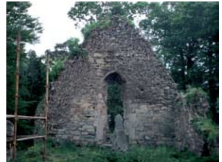
Elevation showing ivy after herbicide treatment
