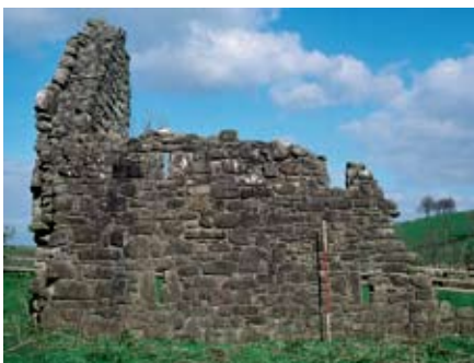
Loose stonework can present a safety hazard
