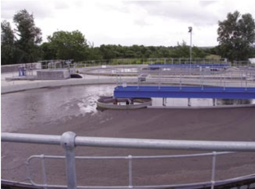
Figure 1: Primary Settlement Tanks at Strabane WWTW
