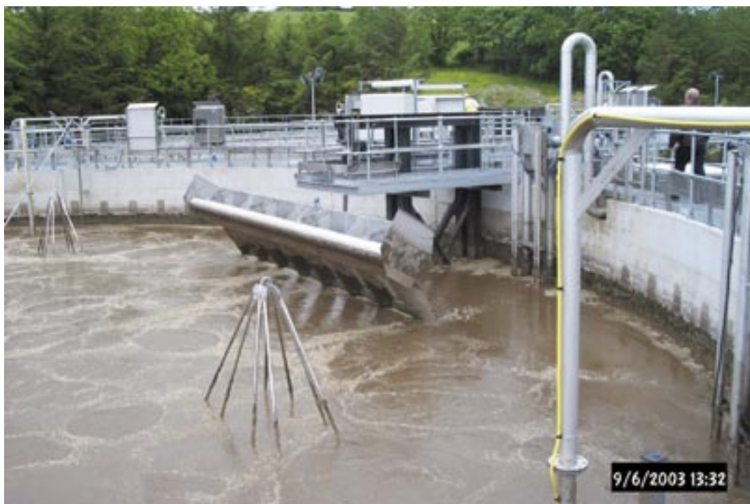
New Sequencing Batch Reactor (SBR) at Banbridge
