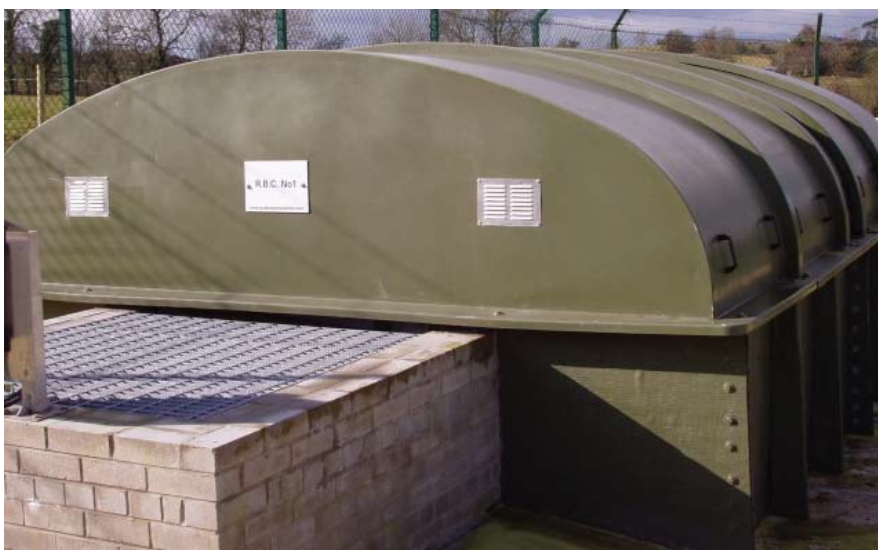
Figure 7: Rotating Biological Contactor (RBC) at Rock WWTW
