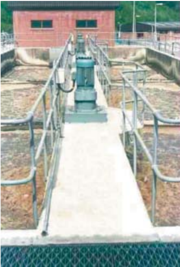
Aeration tanks at Newtownbreda WWTW
