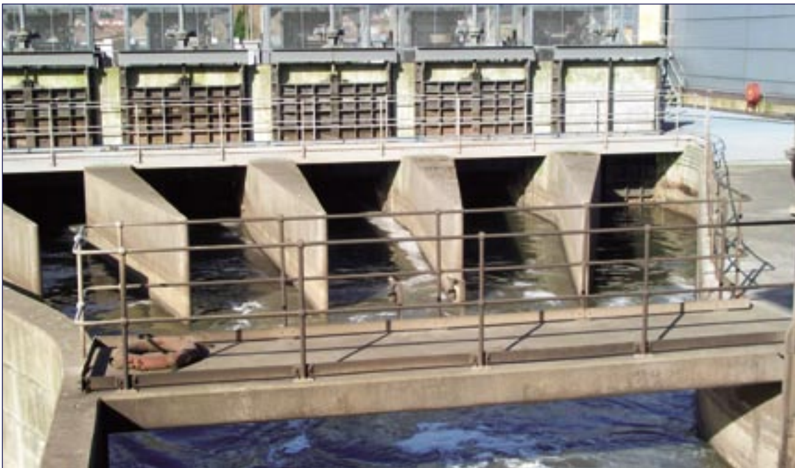
Figure 8: Inlet Screens at Belfast WWTW
