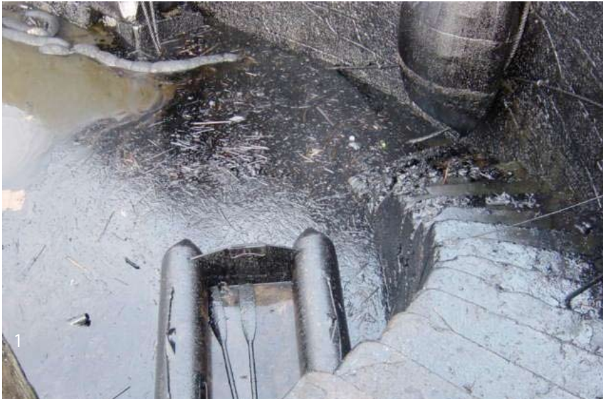
1. Impact on Dock Due to a Significant Oil Spill
