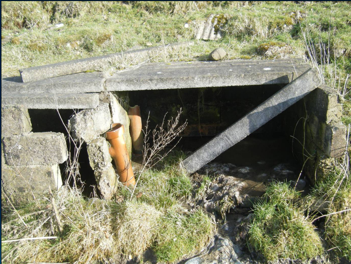
Defective septic tank
